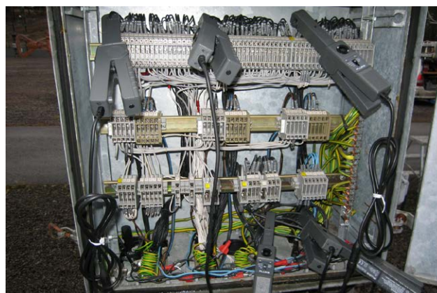
Figure 3 Control cabinet with current clamps
